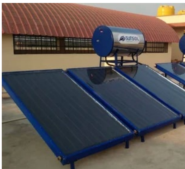
Solar powered water heater
