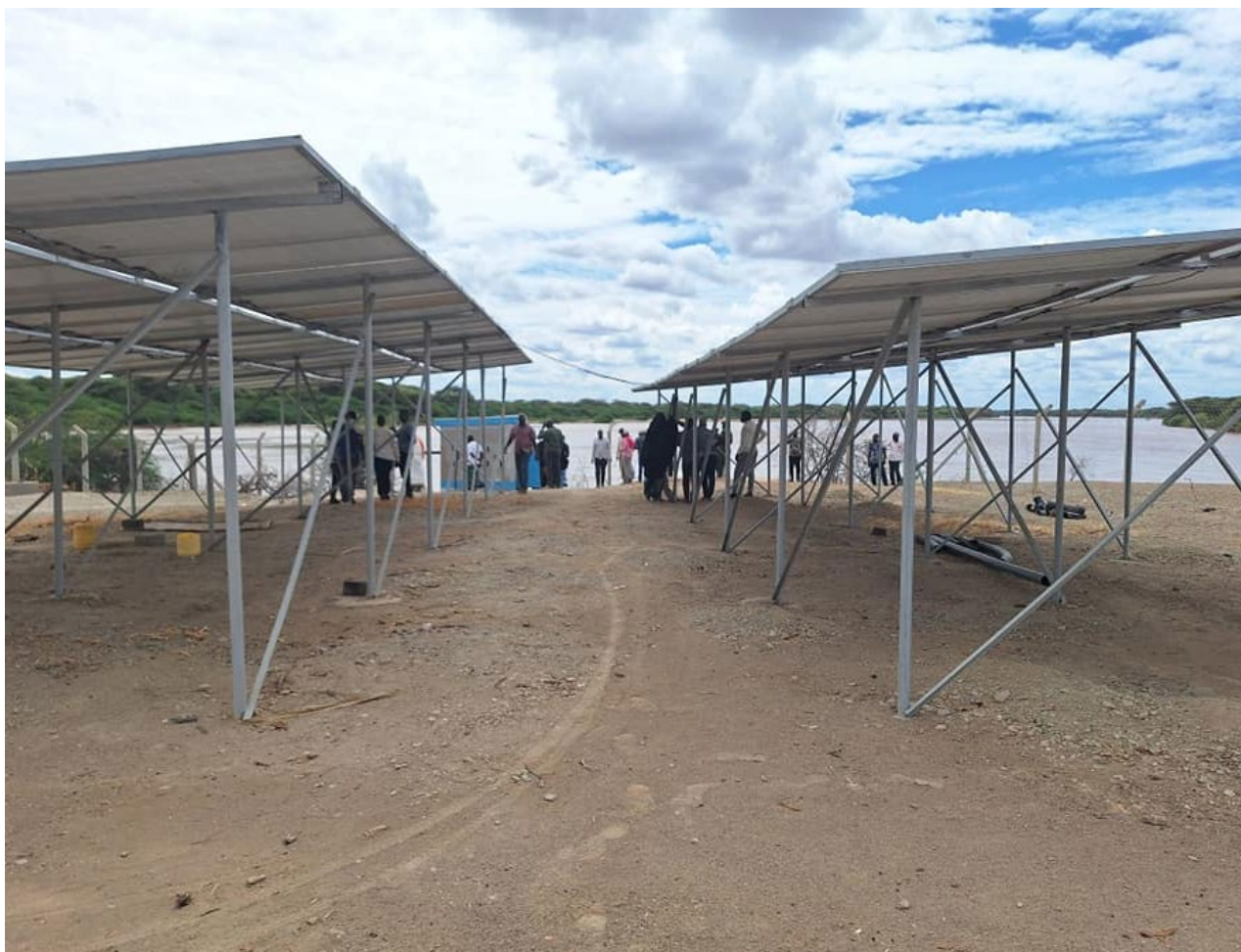
Solar powered water pump in Tana River County
