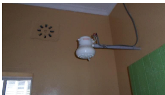
Figure 5.5: Hot water shower
