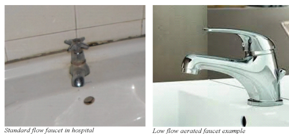
Figure 5.4: Faucets installed in County Buildings
