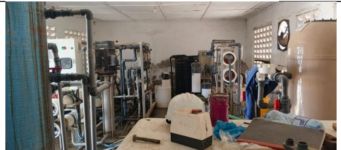
Figure 8 Interior of the solar desalination system, including operational components
