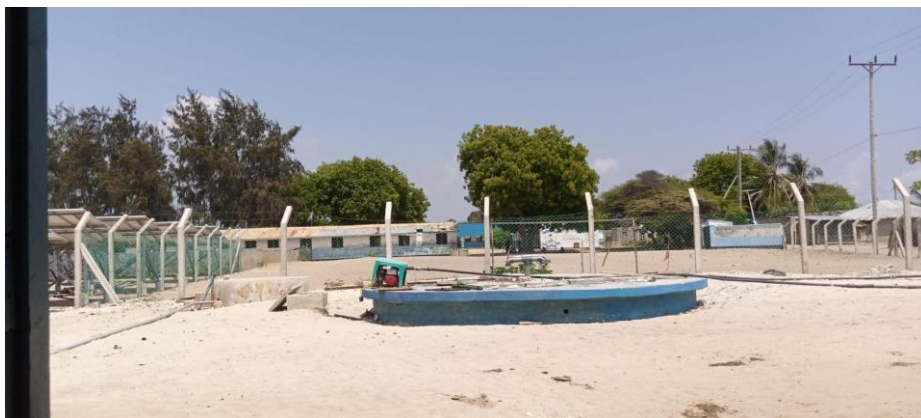
Figure 2A concrete sump tank at the Kiunga Solar Desalination Plant used to support storage and regulated distribution of treated water to households and institutions
