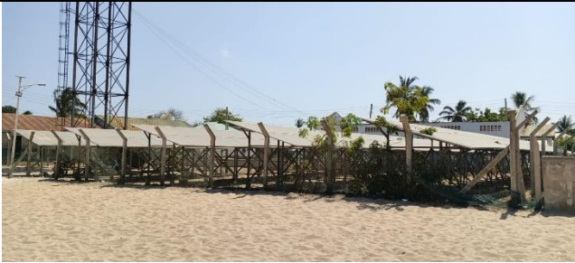
Figure 11 A photo of Kiunga Solar desalination plant
