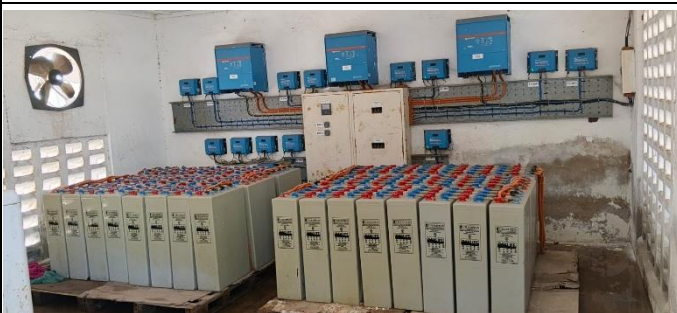
Figure 7 Interior of the solar desalination system, including batteries and operational components
