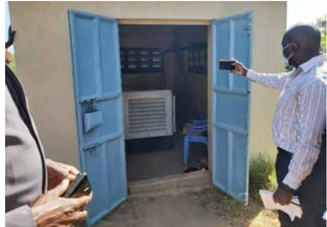
Kwa Mbila Dam water pump is operated by a PMC member
